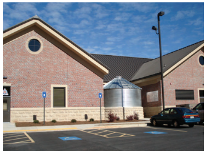
The Emergency Operations Center in Douglas County collects and stores rainwater.
