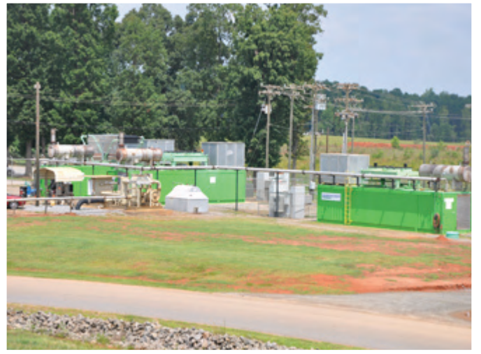
Catawba County Landfill Gas-to-Energy Facility
