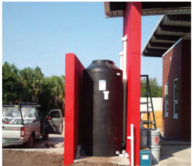
This roof in St. Petersburg, Florida is designed to collect and store rainwater.
