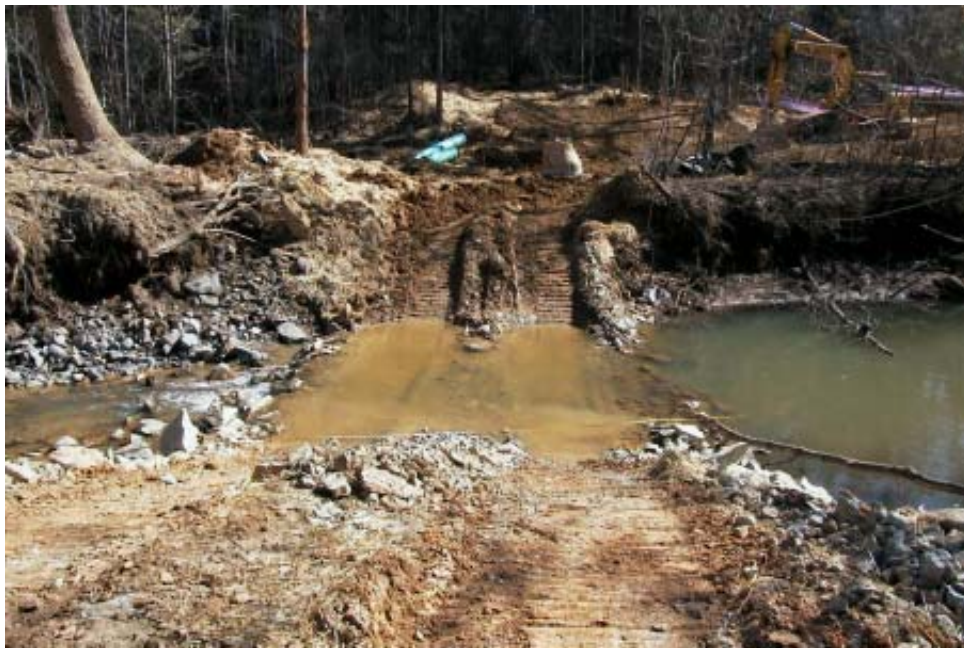
Construction site on Westbrook Creek, Cobb County; an example of a stressor to imperiled fish species in the Etowah. Photo by Jesslyn Storey.
